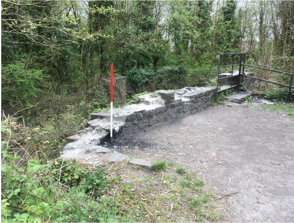
Fig 2. The eastern wall of the woollen mill showing damage to stonework by vandalism (28/04/21)
