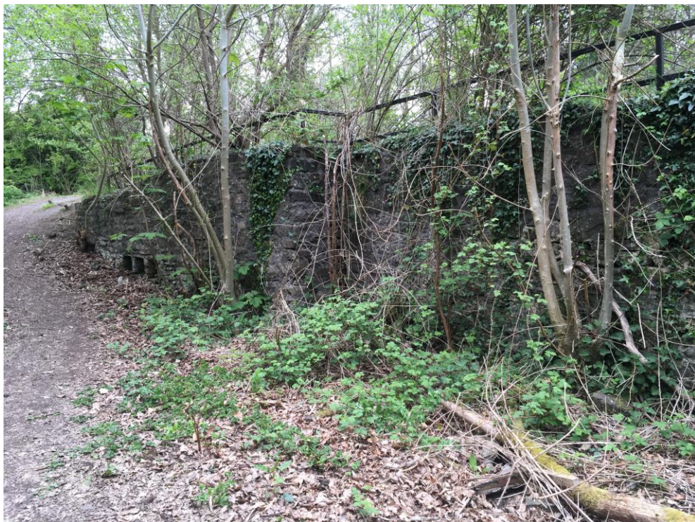
Fig. 3. Invasive vegetation & trees growing out of stonework of retaining wall (28/04/21)
