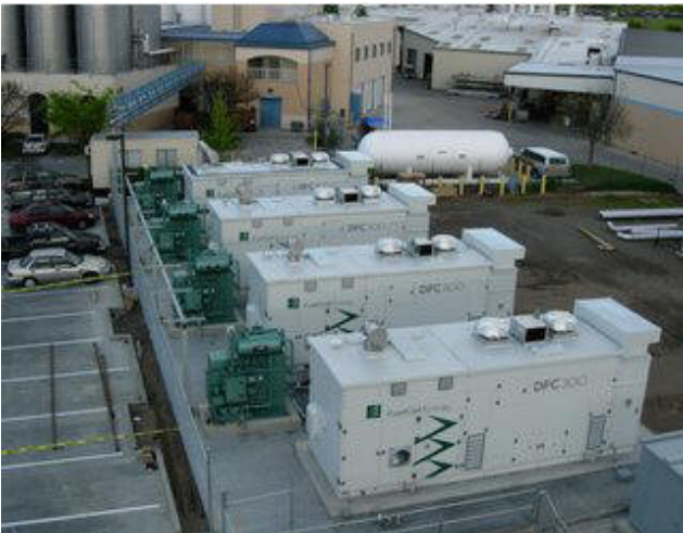
Figure 2.13: IMW (4x250kW) fuel cell plant, Sierra Nevada, California [Courtesy of SCS Energy]
