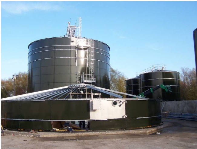
Figure 2.4: Wanlip 1.4MWe anaerobic digestion plant (Bursom, Leicester)
