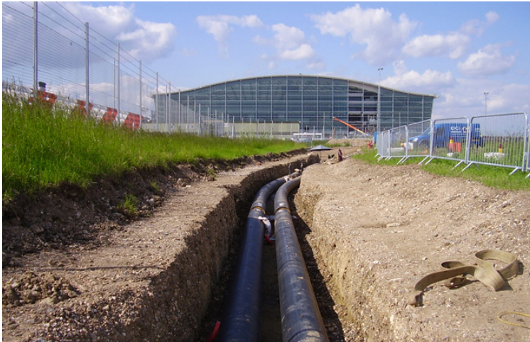
Figure 2.15: Heat main pipework at Heathrow Airport, Terminal 5 [© Vital Energi | www.vitalenergi.co.uk ]
